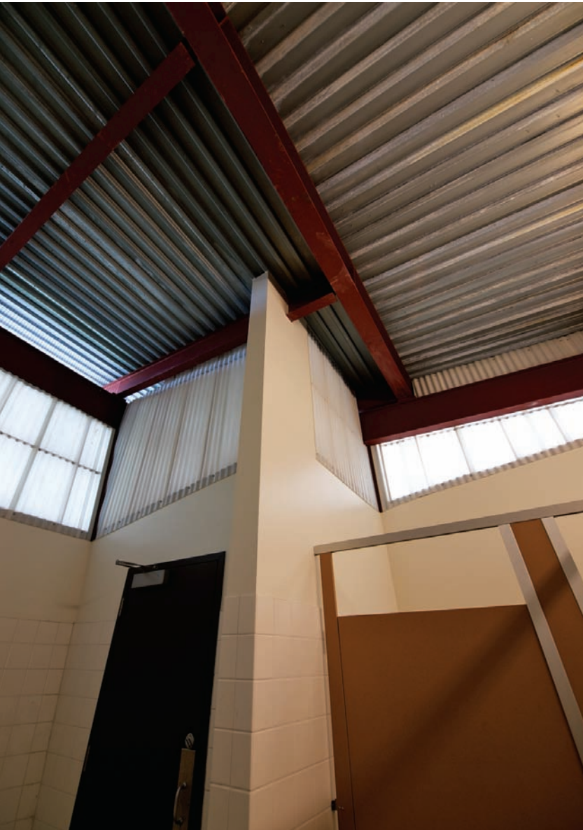
Below: Interior view from within the restroom facility towards the interlaced planes of steel decking and corrugated fiberglass panels at the roof level. The translucent panels help illuminate the restrooms and minimize the need for supplemental light.
